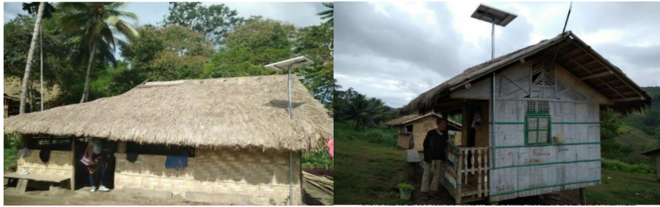
Diagram 8 : Roof-through Pole mounted installations on thatched roof
