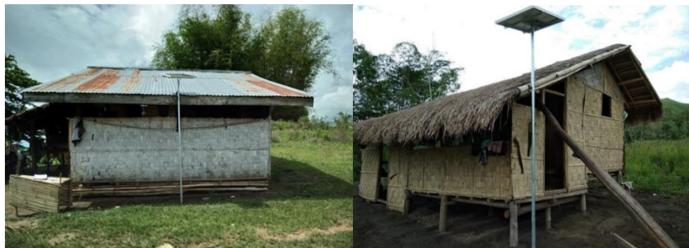
Sample Roof-side Pole mounted installation
